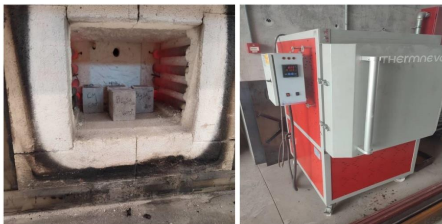
Figure 8. An electric chamber furnace.
